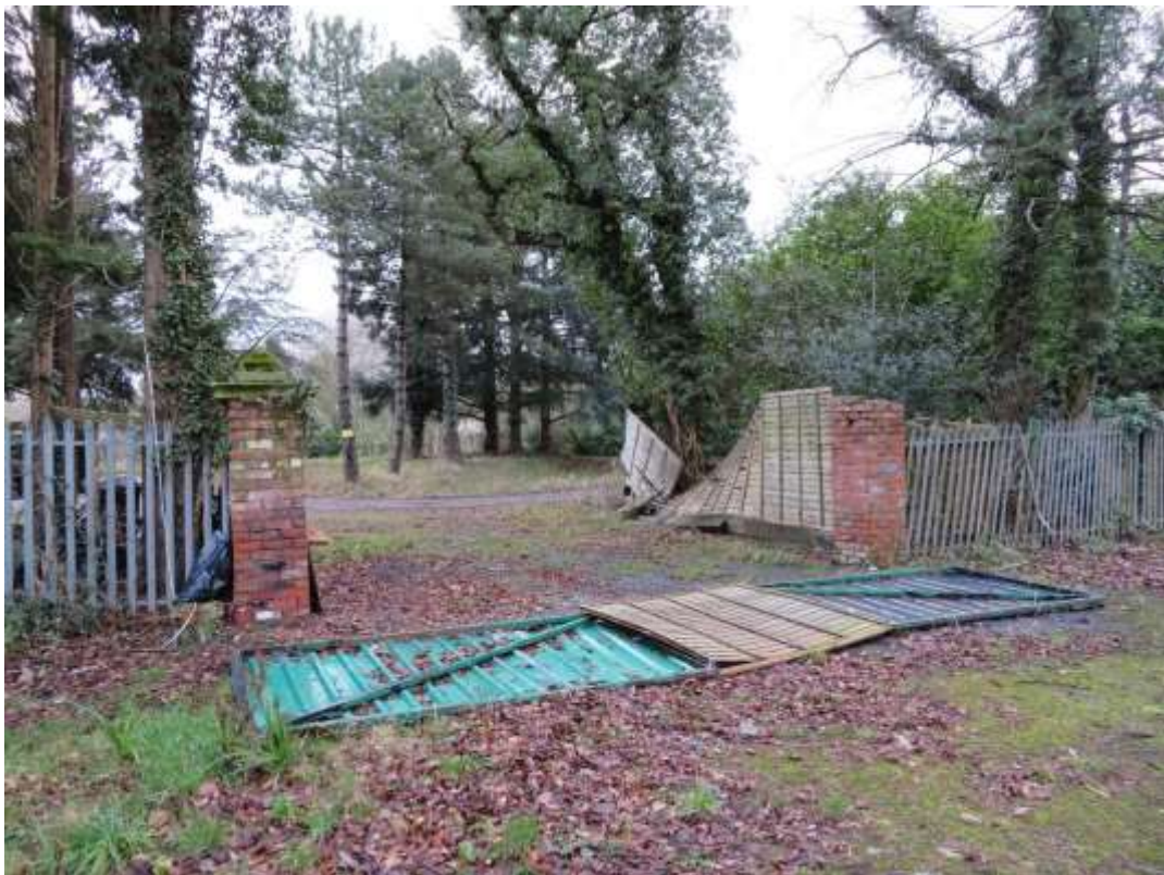
Plate 7 The private gateway created by Samuel or William Cunliffe Brooks to lead onto Brooks Drive. It is currently in poor condition
